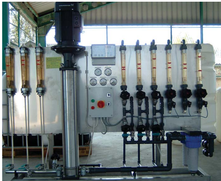
Figure 3. UF-NF-RO pilot plant.
